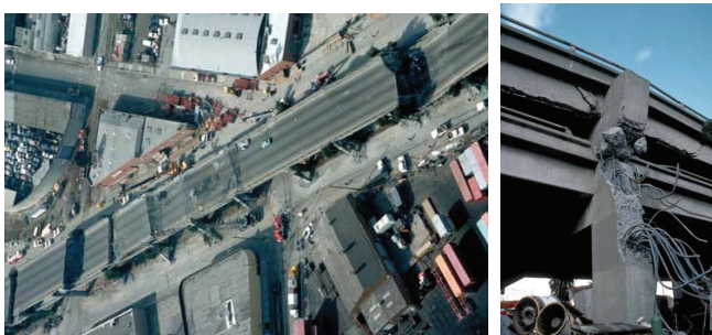
Fig. 1. Loma Prieta, sections of the Cypress viaduct (H.G. Wilshire, U.S. Geological Survey)
